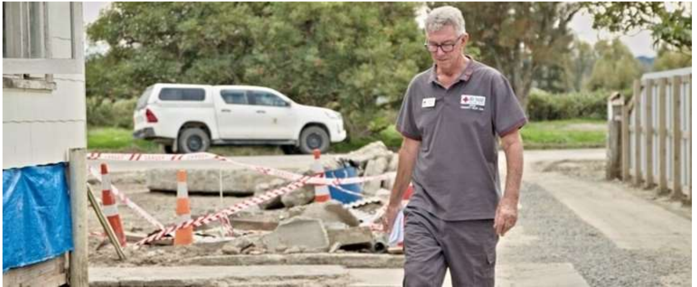
Phil Parker is seen inspecting damage caused by Cyclone Gabrielle in Wairoa.
